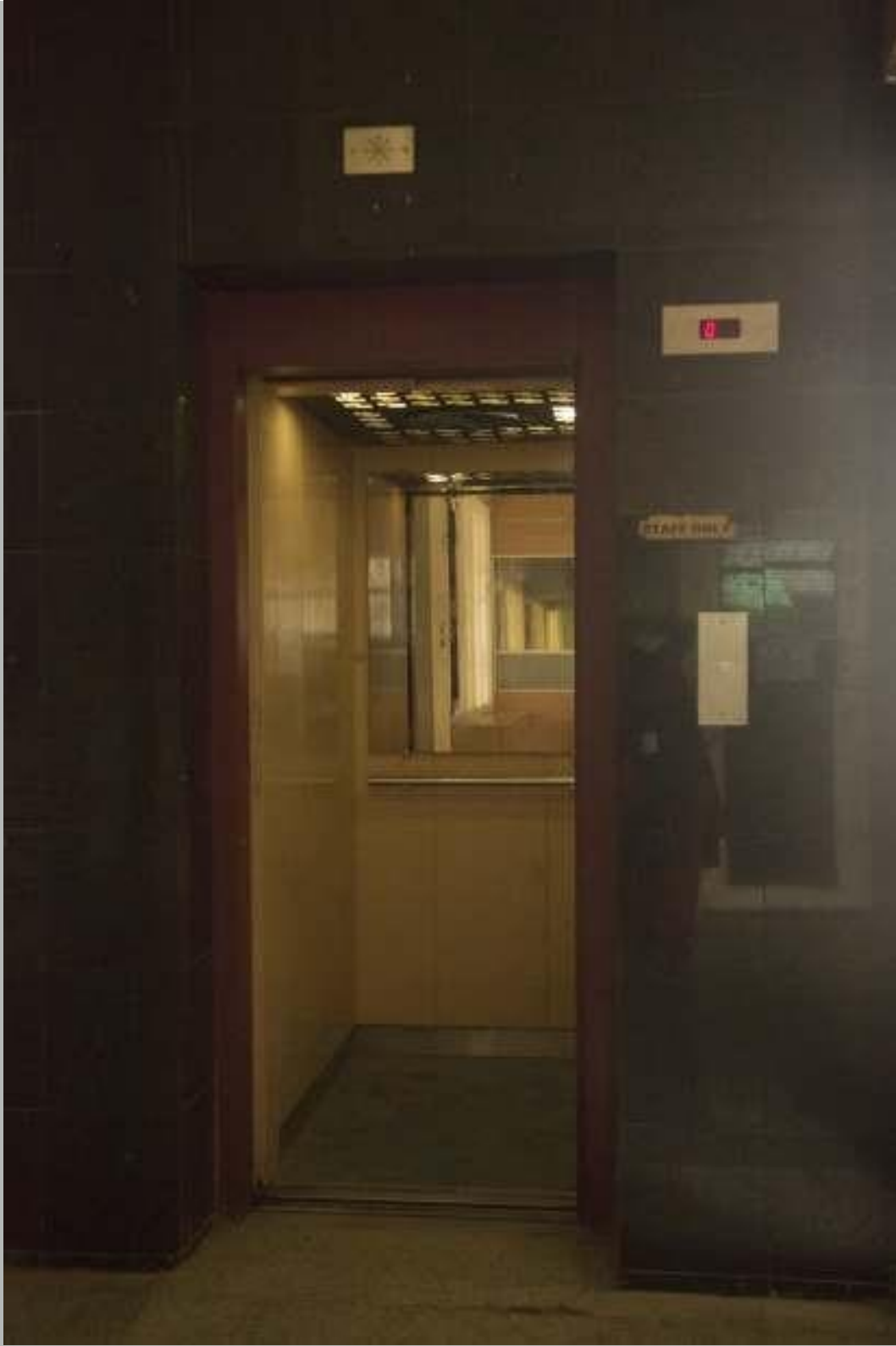
Elevator Facility at St. Francis Block
